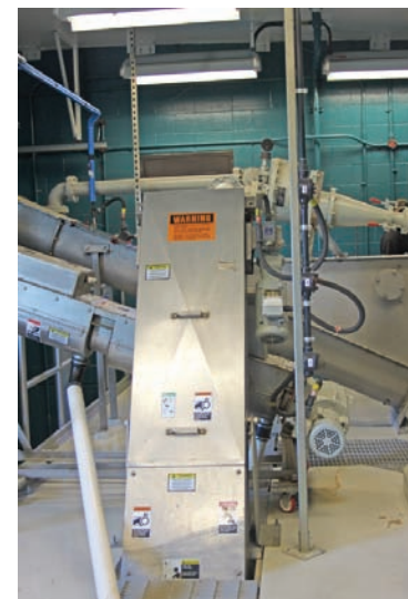
A bar screen system from Siemens is shown in the foreground with the WesTech grit removal system behind it.
